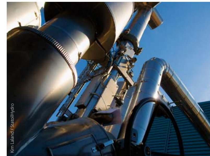
Improved planning with Safran Project at the Kårstø processing plant
